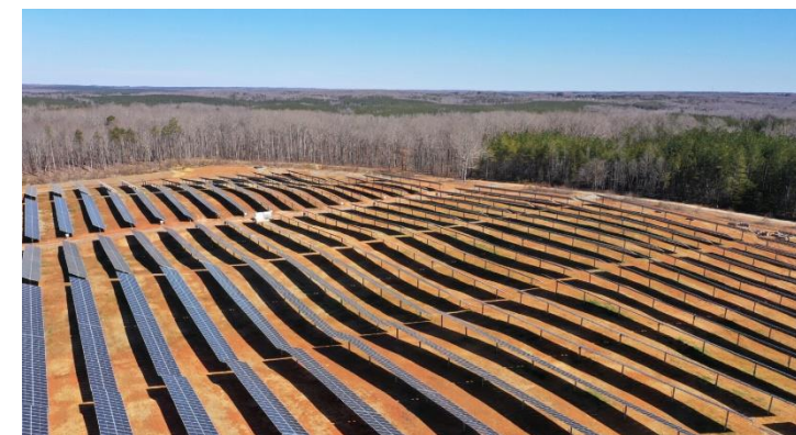
EPC Contractor Virginia – 17 MW
