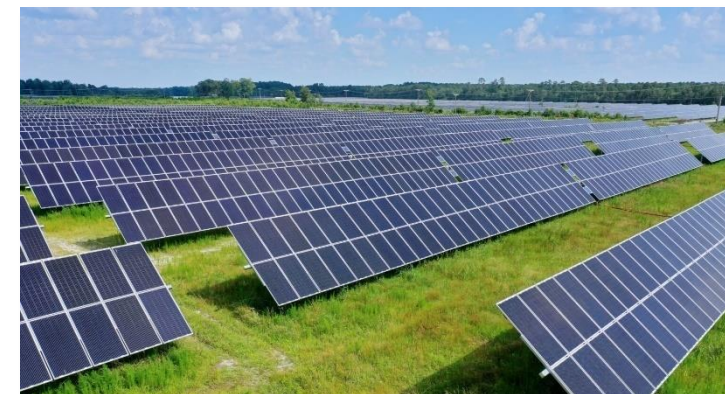
EPC Contractor North Carolina – 112 MW
