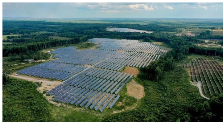
Developer South Carolina – 97 MW
